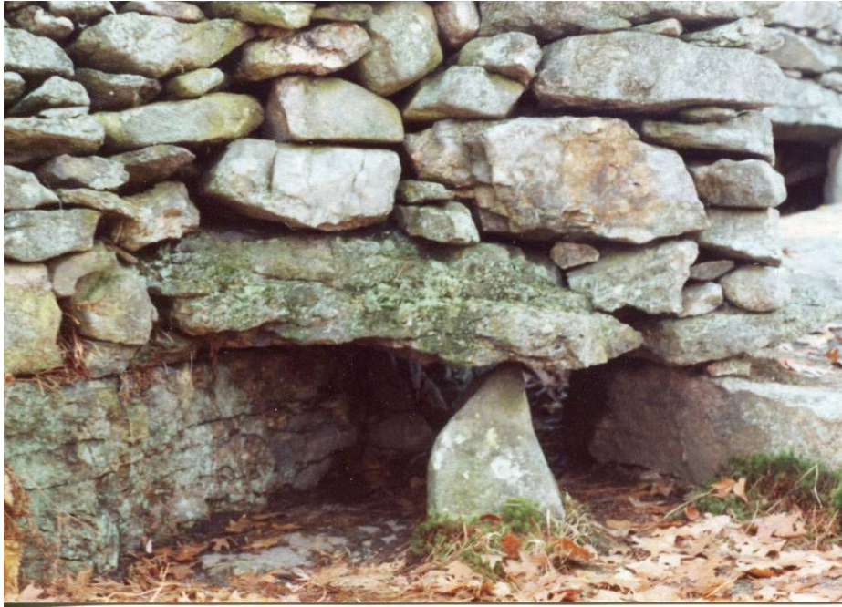
Figure 25 – Close-up of the drain exit under the Half-Circle Enclosure. (Photograph by Mary Gage)
